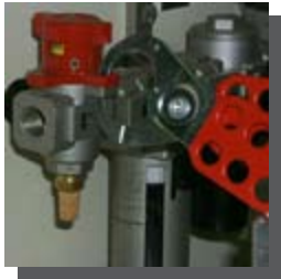
figure 65-1. Main Air Gate Lock-Out
