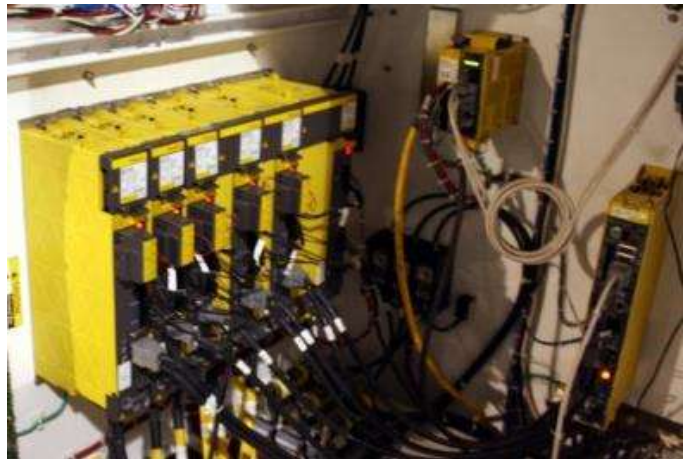
Fanuc Electrical Components (Most reliable control system in the world "average mean" between failures of 10 years)
