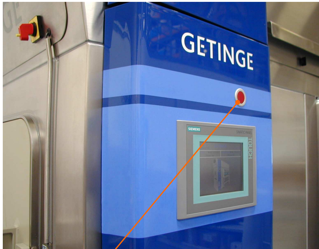
"Emergency aeration" button
