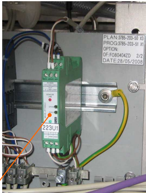
Transmitter (installed on the PLC plate at the top)
