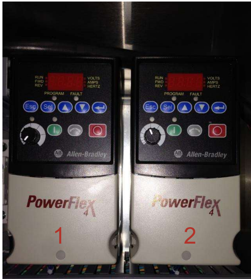
Figure 12 Variable Frequency Drives (VFD's): #1 for main conveyor motor and #2 for seamer motor
