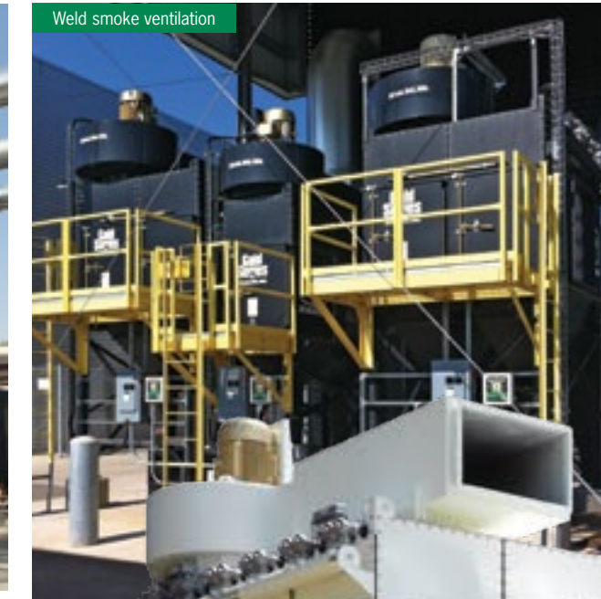
Weld smoke ventilation
