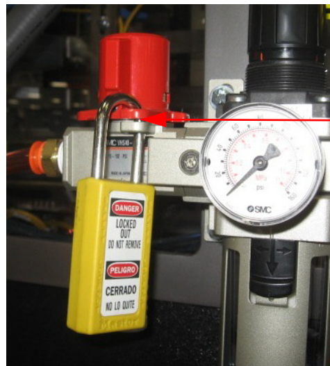
Figure 1 - 4 Pneumatic Lock Out
