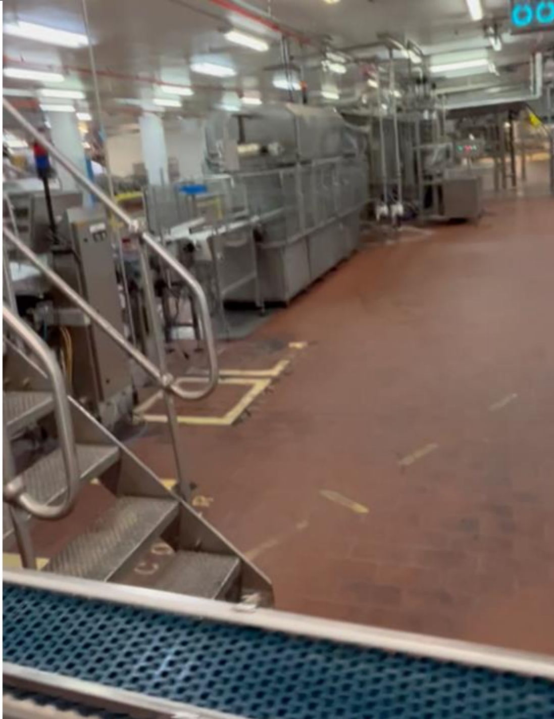
Conveyor turns through 2No. 90 Degrees and heads for x ray section
